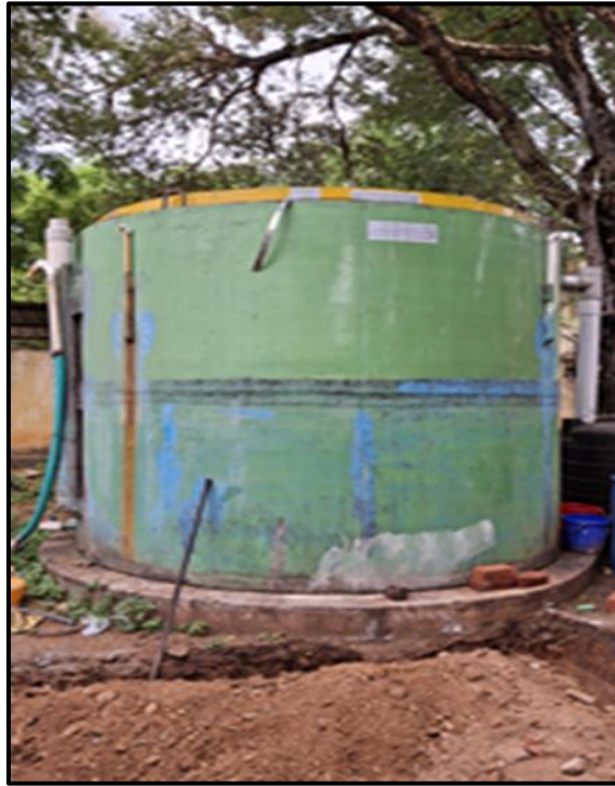
Biogas Facilities were observed in the campus
