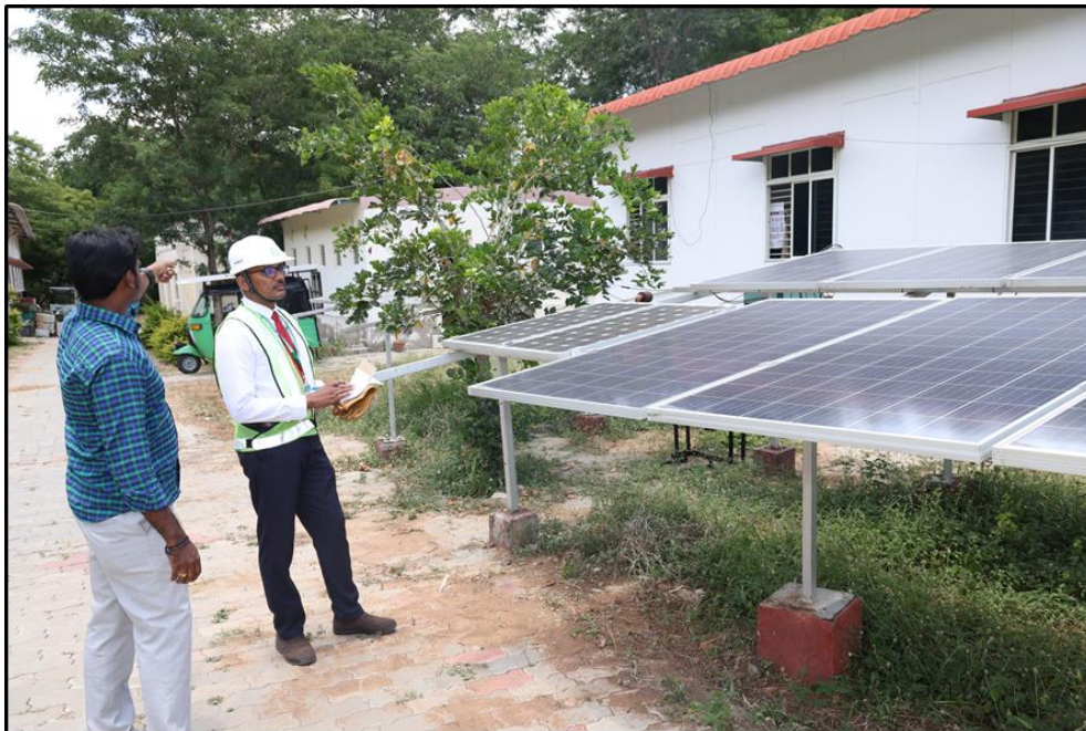
Solar panel observed in the campus
