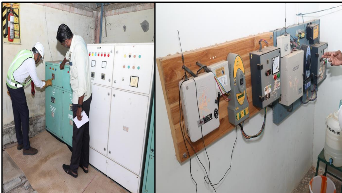
Energy conservation facilities observed in the Campus
